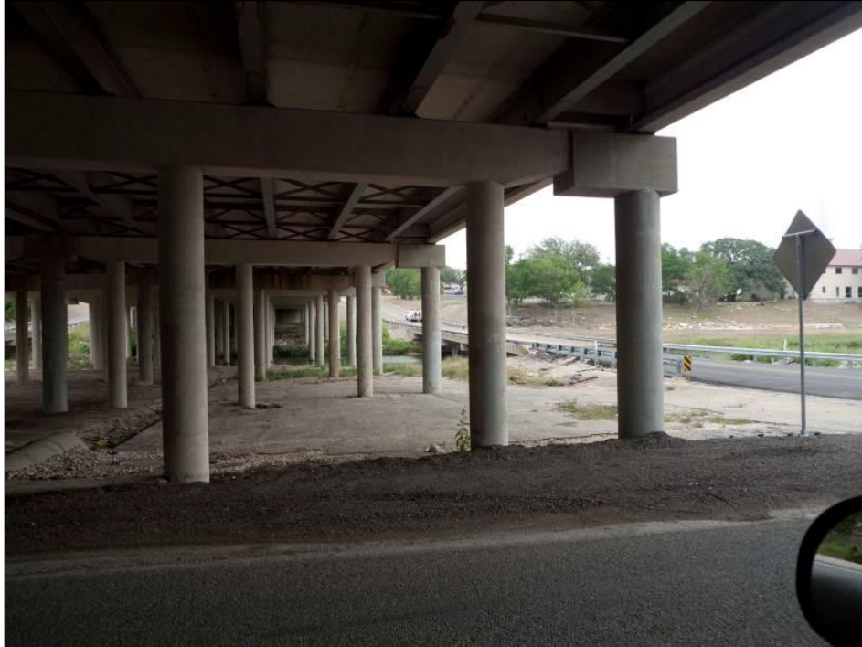
Figure 1.3. The underside of Salado Creek bridge in Bell County, Texas, showing the existing main-lane bridge (left side), currently occupied by bats.
