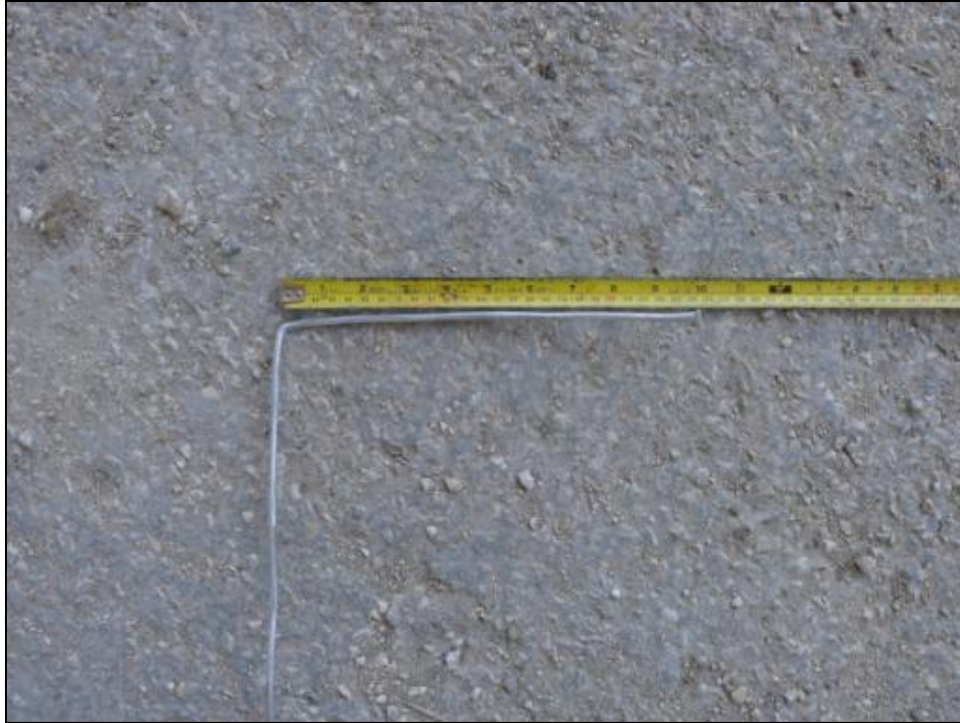
Figure 2.4. The width of the T at the top of the gap at Lampasas bridge, Bell County, Texas, varied along the length of the bridge. Stiff wire of varying known lengths was used to estimate the width at each meter.
