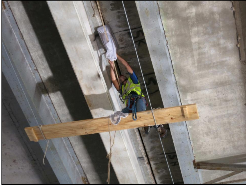
Figure 3.7. Trolley systems were installed under both the Lampasas and Salado bridges, Bell County, Texas, to allow us to access more of the gap than ropes alone.
