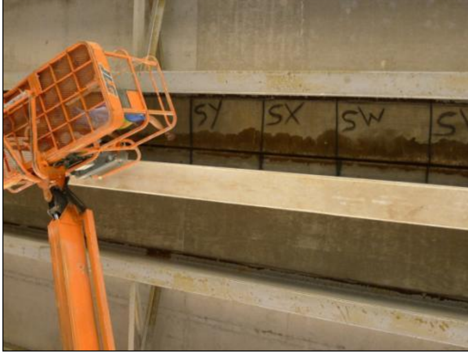
Figure 2.1. Each linear meter of the gap at the IH 35 bridges over the Lampasas River and Salado Creek in Bell County, Texas, were assigned an alphabetical identifier, which was semi-permanently marked directly on the underside of the bridge using spray paint. Also visible in the image are stains from bat urine.
