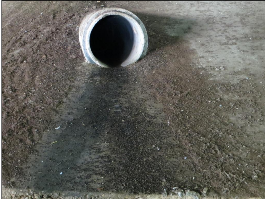
Figure 4.10. Storm water outfall under the south side of the main lanes of the Lampasas bridge, Bell County, Texas. Note the newer guano deposits (black) that have accumulated since the last rainfall event and the older, thicker guano deposits (brown) that are not washed away by storm water.
