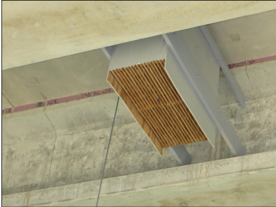
Figure 2.8. An installed bat house at the Lampasas bridge, Bell County, Texas, showing rope access for future monitoring.
