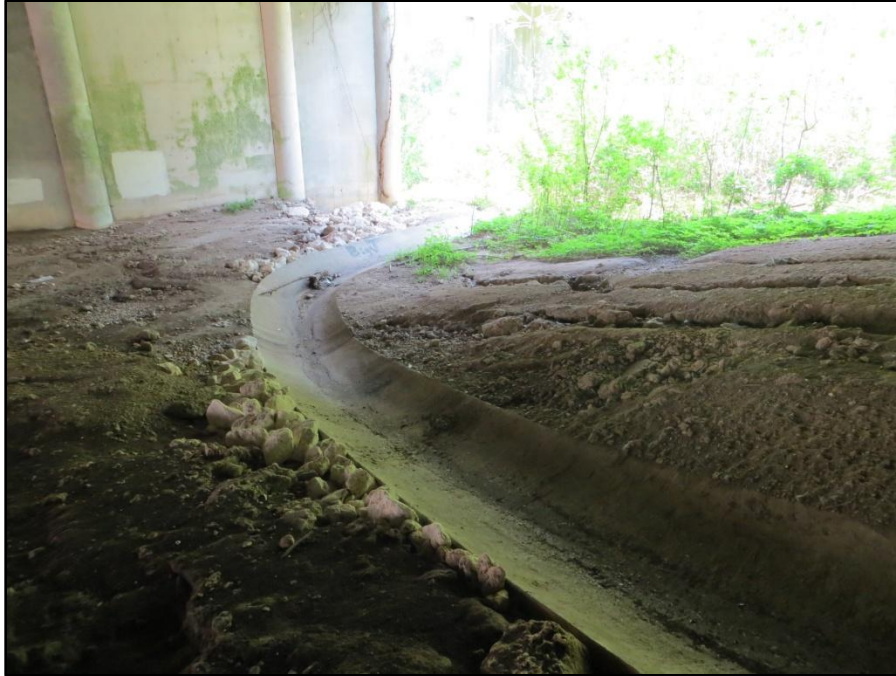
Figure 4.5. Concrete drainage gutter that conveys storm water from the outfall underneath the north side of the Lampasas bridge, Bell County, Texas. Bat guano can be seen in the gutter.
