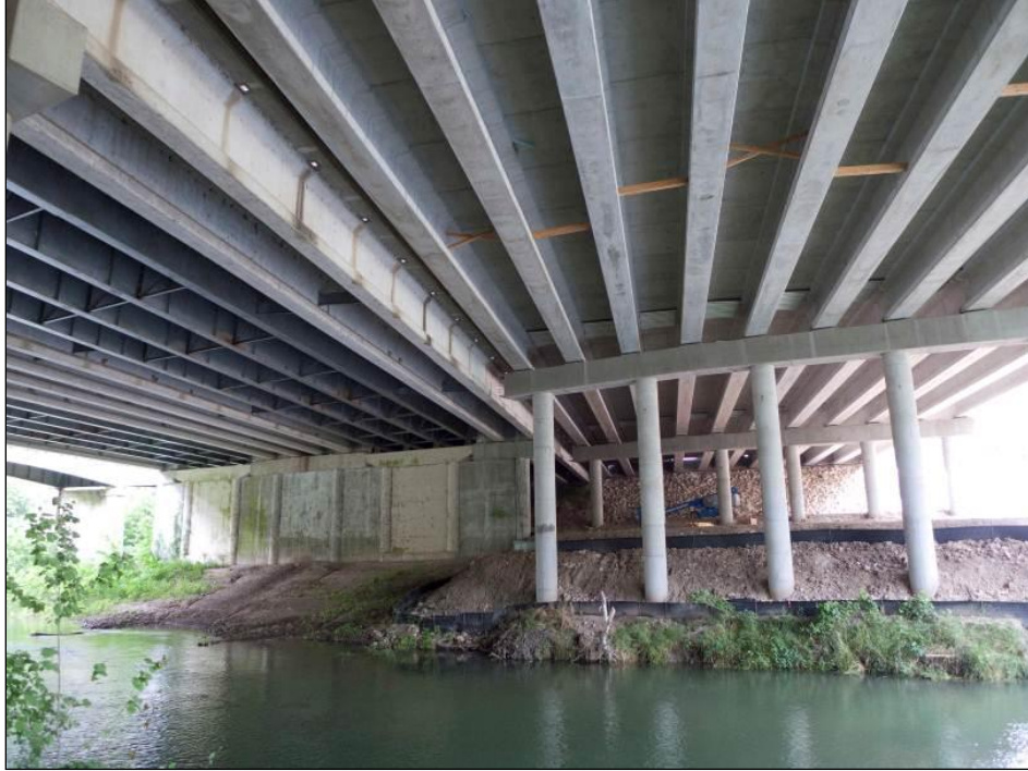
Figure 1.2. The underside of the Lampasas Bridge in Bell County, Texas, showing the existing main lane bridge (left side) currently occupied by bats. The area to the right side of the photograph shows the new main lanes currently under construction.
