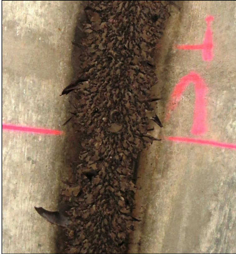
Figure 3.2. Bats stacked several deep into the gap and bulging out of the gap during periods of high occupation at the Lampasas bridge, Bell County, Texas.
